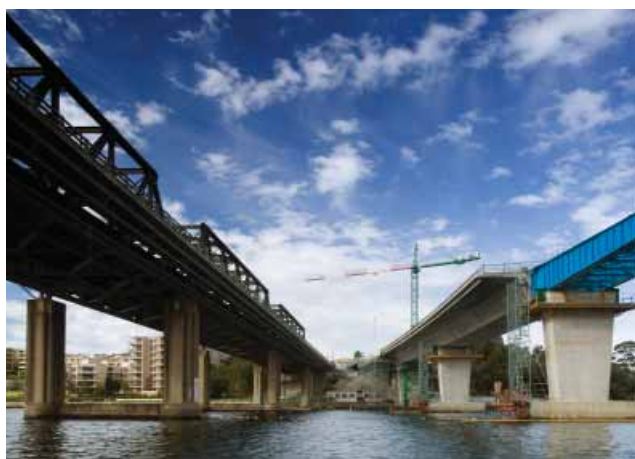
Construction of the new bridge adjacent to the existing bridge over Iron Cove Bay, June 2010.
