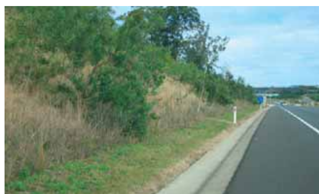
Vegetation growth on the Bonville Bypass, Pacific Highway, in June 2010, just two years after opening.
